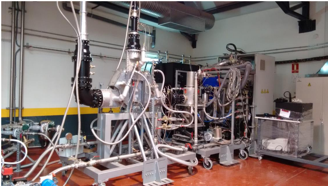
Fig. 12. High power RF source of the CIEMAT High Power RF Laboratory
