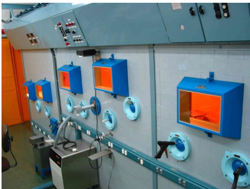
Fig. 26. Radioactive facility for mechanical characterization. Outside
